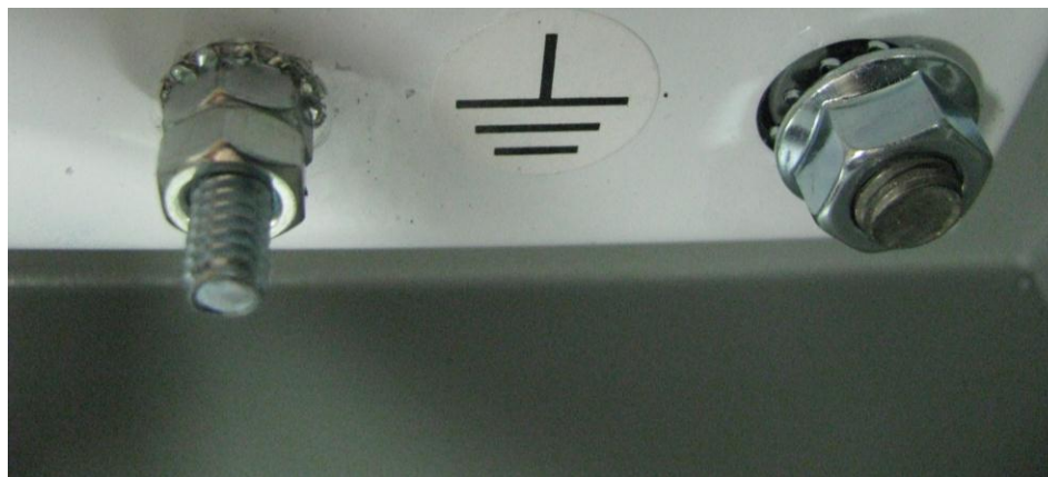
Figure 5. Earth Ground Terminal.
